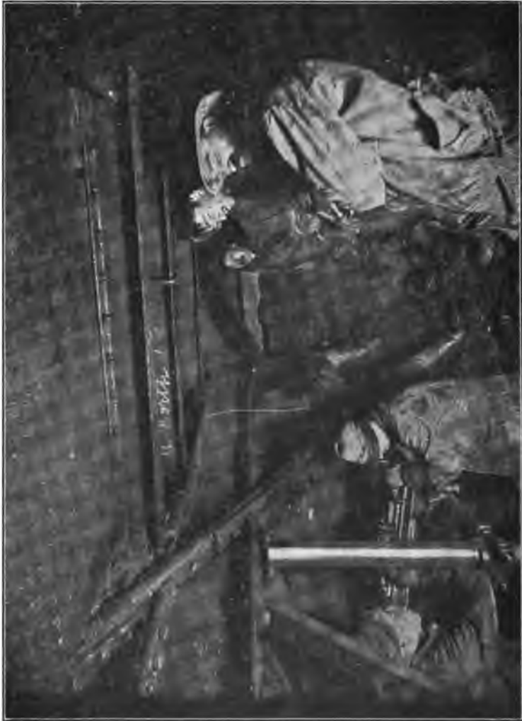
EXCAVATING UNDER TEMPORARY COVER IN FRONT OF SHIELD, HUDSON RIVER TUNNEL, NEW YORK.
