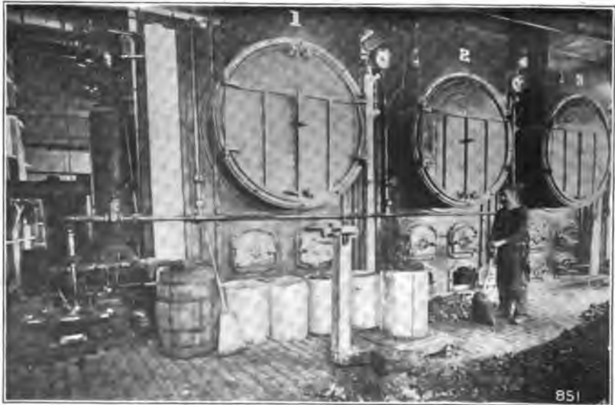
FIG. 2—BOILERS FOR COMPRESSOR PLANT, SECTION "C," BOSTON TRANSIT COMMISSION.
