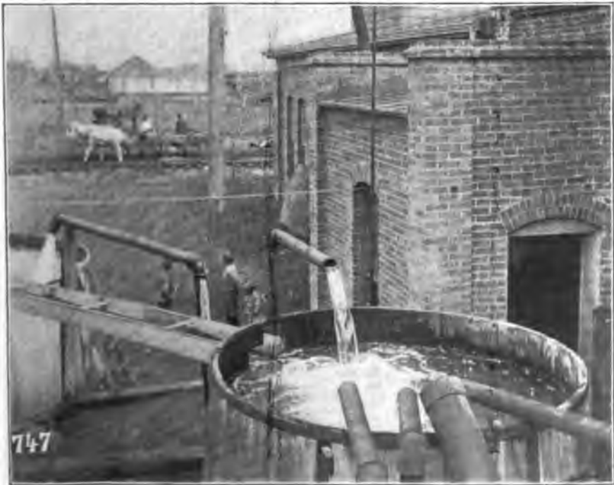
AIR LIFT PLANT. CAPACITY 600,000 GALLONS IN TWENTY-FOUR HOURS.
