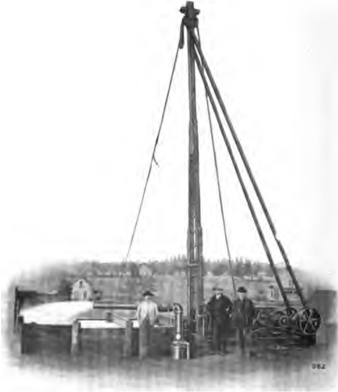
SOUTH TACOMA AIR LIFT PLANT.
