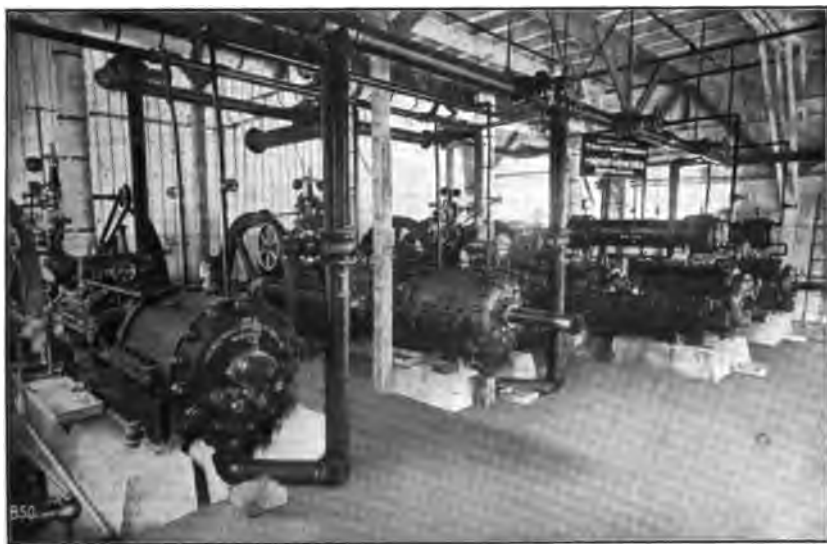
FIG. 1—COMPRESSOR PLANT, SECTION "C," BOSTON TRANSIT COMMISSION.
